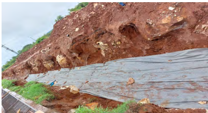
Figure 3: Showing excavation of infiltration drain system with geotextile layer at the base.
